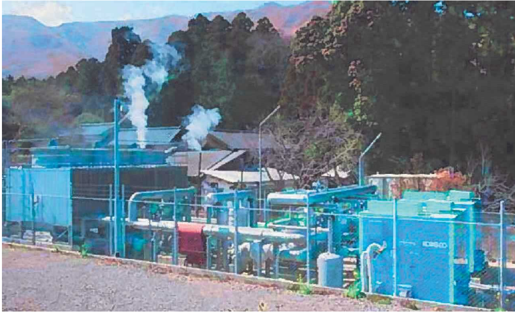
Figure 3-8 Yuyama Geothermal Power plant
