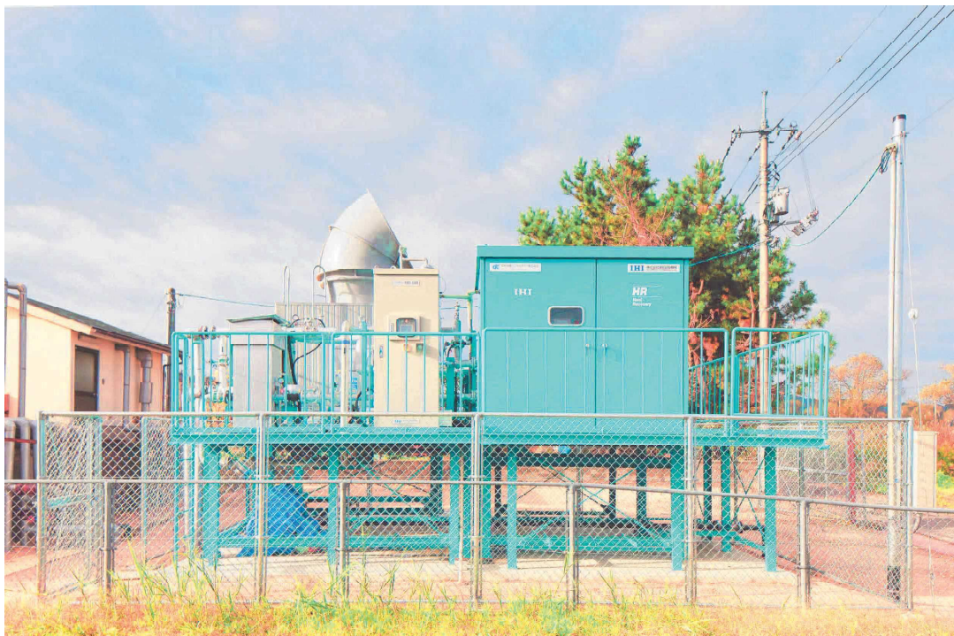
Figure 3-9 Yurihama Geothermal Power plant
