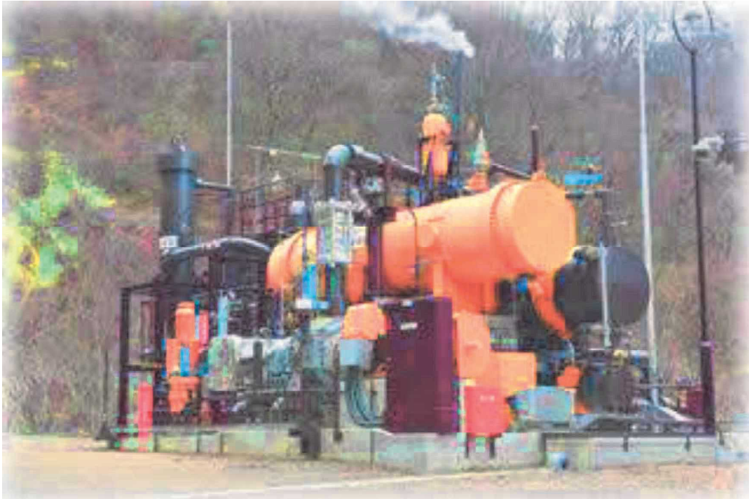
Figure 3-10 Tsuchiyu Onsen #16 Source Binary Power plant
